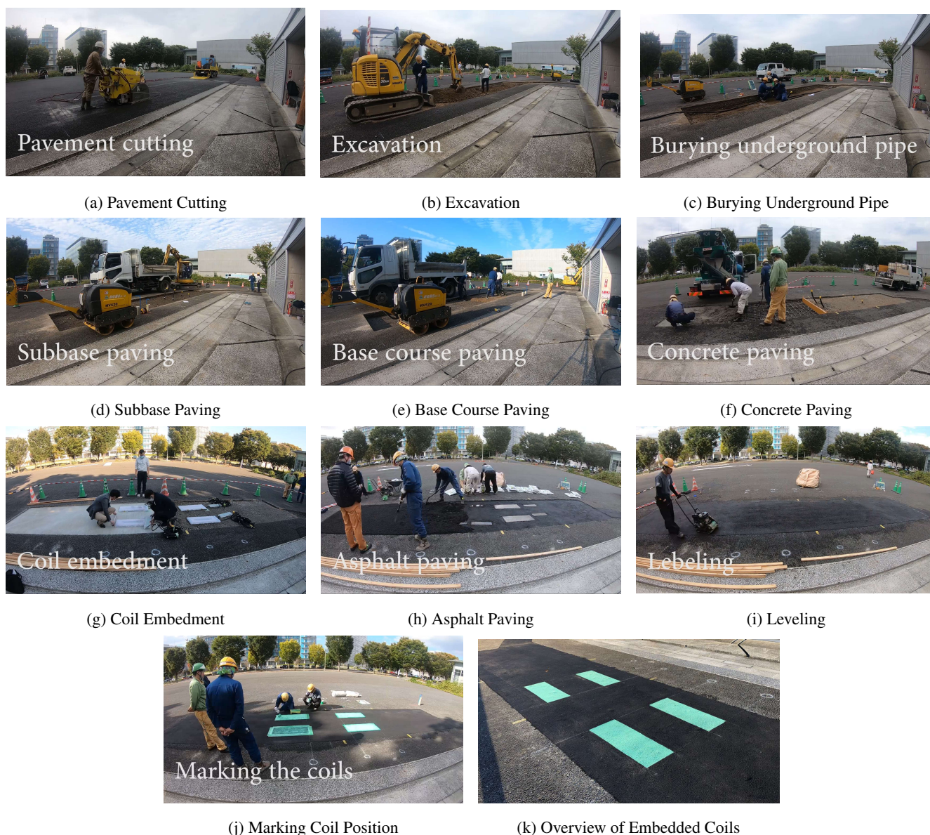
図 5: 給電コイルの埋設工程 Fig. 5. Procedures of Road Construction for Transmitter Coils
